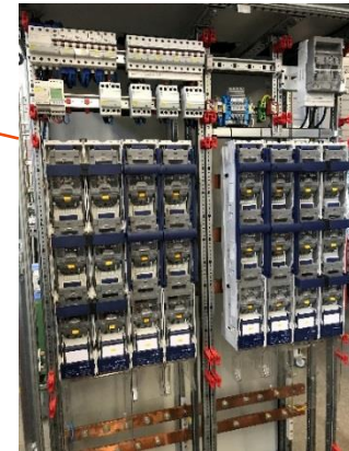
Main distribution board
